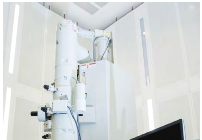
Wall Mounted Chilled Tile Installation
