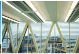
65 Southwark Street London, UK - 2012 Active Multiservice
