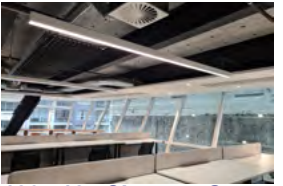
183 - 185 Clarence Street Sydney, AUS - 2020 Active & Passive Chilled Beams
