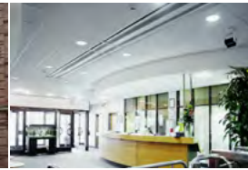
British Gas Manchester, UK - 2000 Active Chilled Beams
