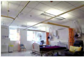
Royal Sussex Hospital Brighton, UK - 2002 Active Chilled Beams
