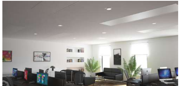
EFW Panels Recessed into Plasterboard Ceiling
