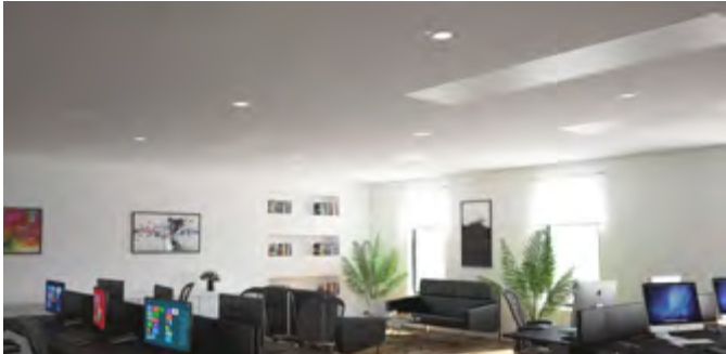
EFW Panels Recessed into Plasterboard Ceiling
